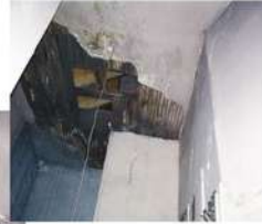
Leak damage to the right of the Altar area
